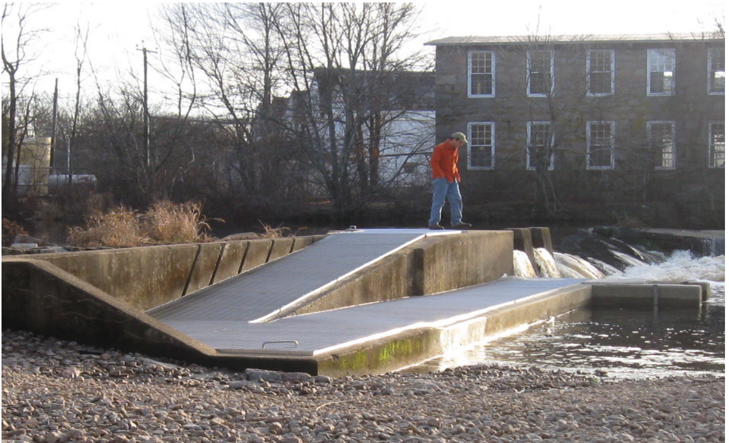
Chris Fox inspects the canoe portage and fish ladder on Bradford Dam after flooding event. Photo: WPWA.
